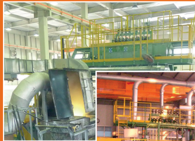
Channel melting furnace
